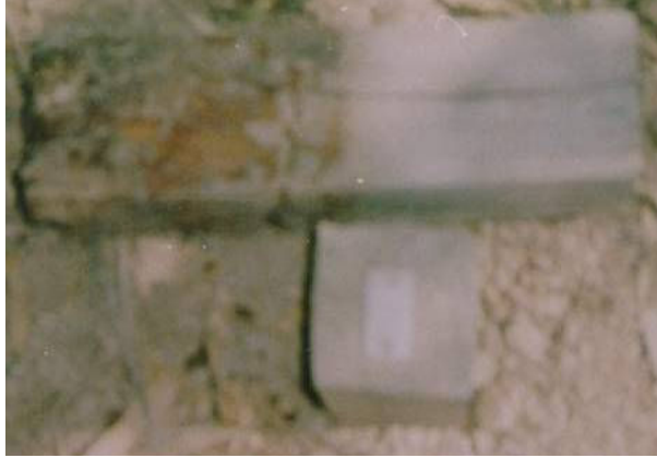
Fig 9-In control samples of E. camaldulensis , the attack by termites started after 36 month, then the grade No. reached to 6.8 after 118 month installation in Mishmast station
