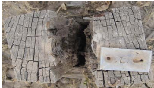
Fig 17– Inside the ground part of control sample is attacked by termites
