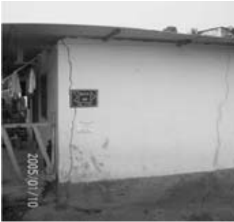
Figure 3: Fissurations of the houses.
