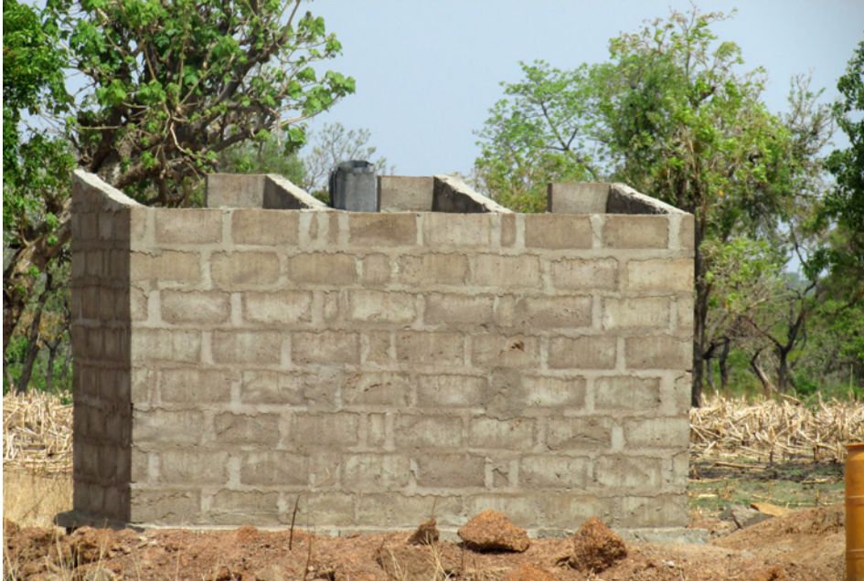
Photo 7.17: A toilet under construction on land of which Sanda does not have “ownership”
