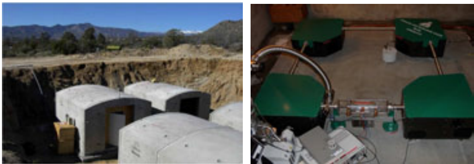
Figure 26. The ring laser vault under construction at the Pinon Flat (Ca) observatory and the GEOSensor installation in one of the chambers.
